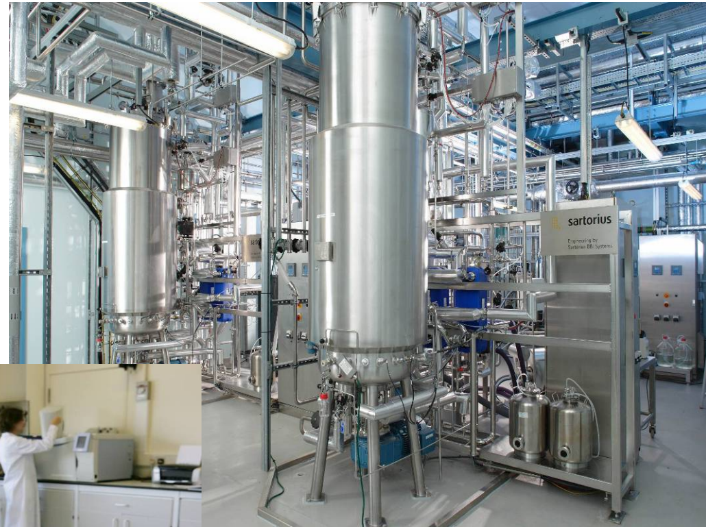
National Industrial Biotechnology Facility
